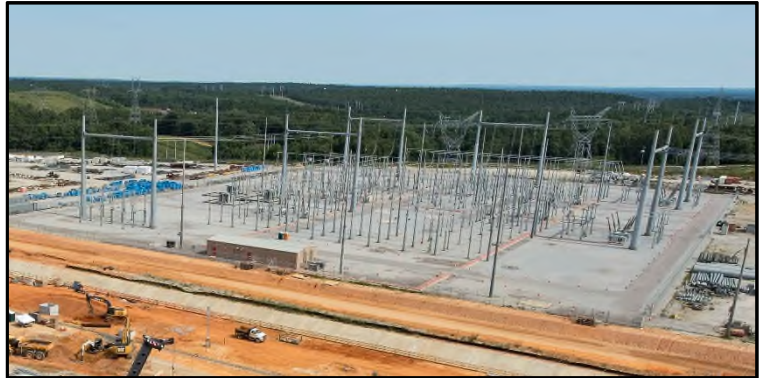
Photo 10 – 500 kV High Voltage Switchyard
