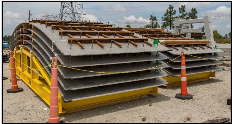
Photo 1 – Unit 3 CB20 PCS Tank Panels
